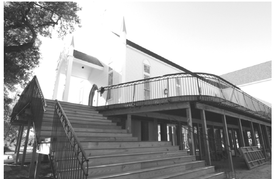
Progress at Trinity Church, which is expected to be completed in March.
