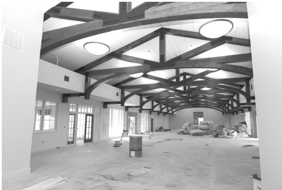
A sneak peek inside the new library, still under construction. Photo by Ron Daley.
